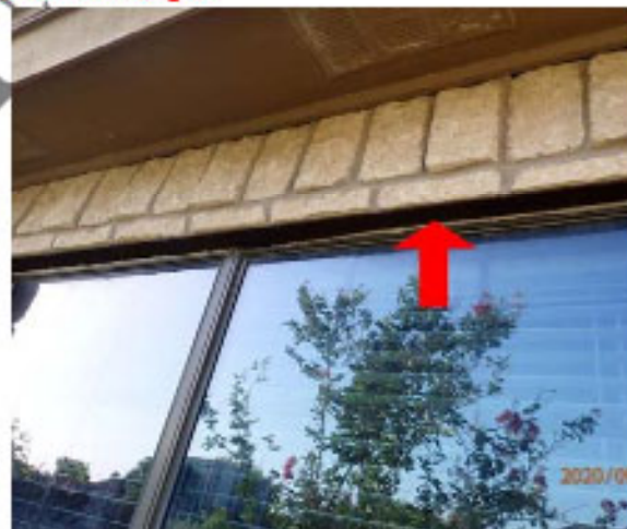
Window Lintel should be painted to prevent rust.
