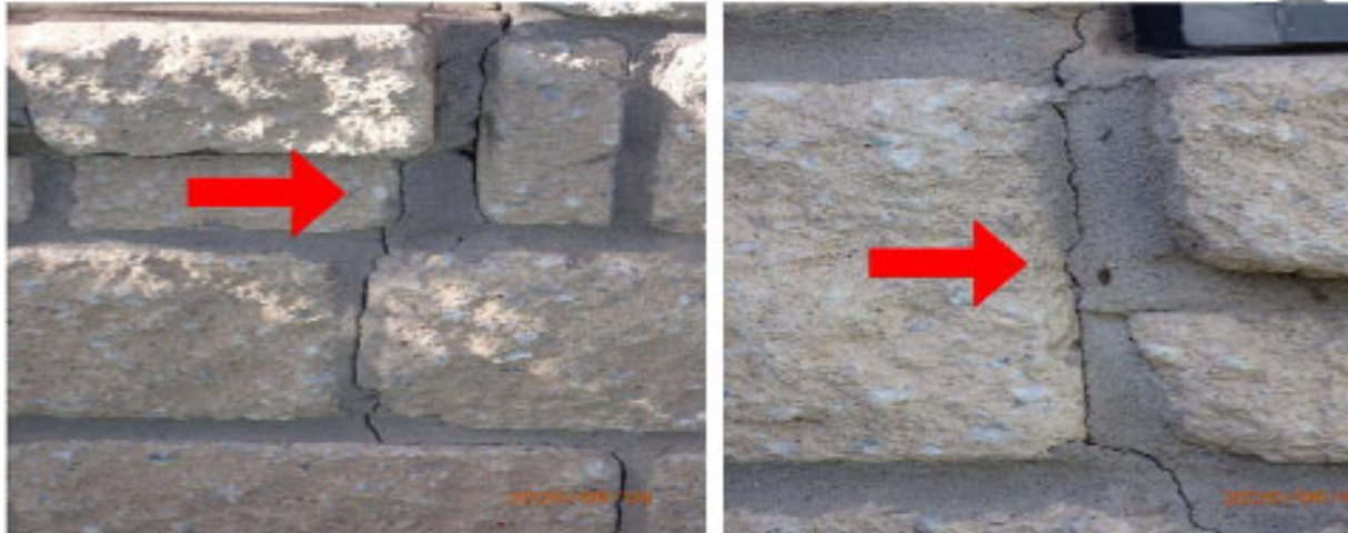
Minor cracks were noted.
