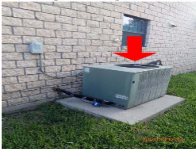
Outside condensing unit.
