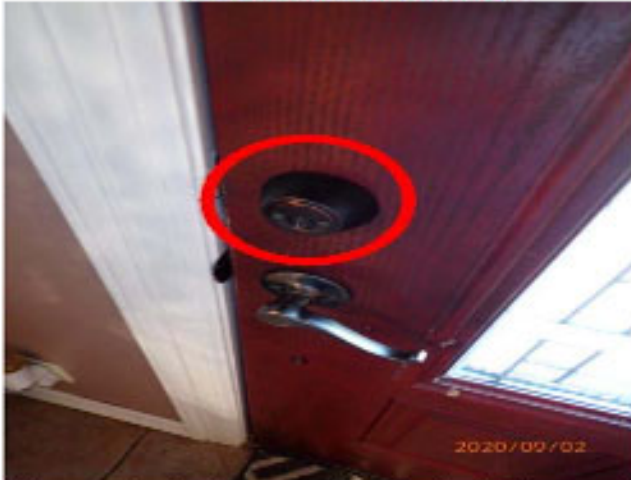
All egress door hardware should be single cylinder.
