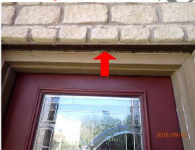
Window Lintel should be painted to prevent rust.
