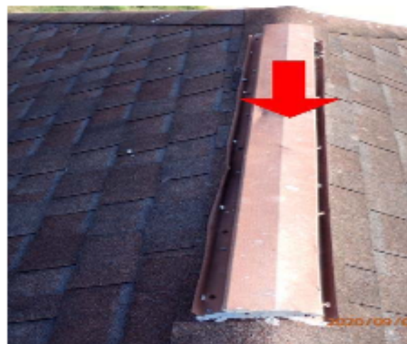
Nail heads are exposed at the ridge.
