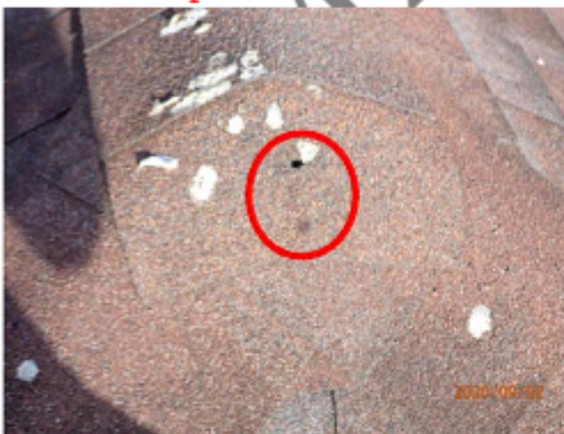
Nail heads are exposed at the ridge.
