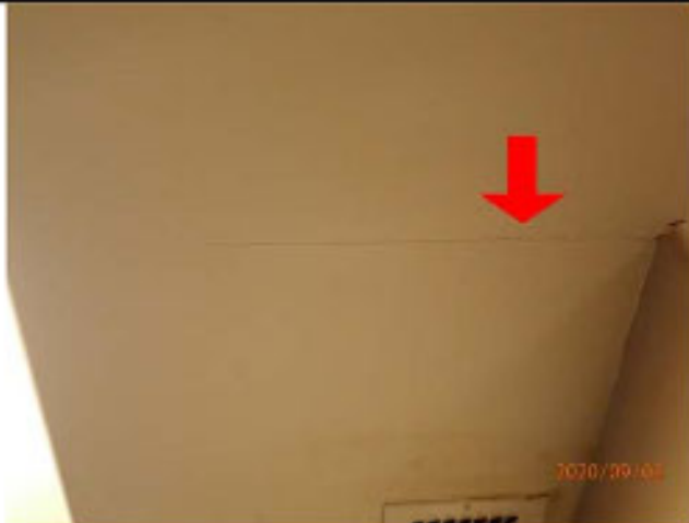
Minor cracks were noted on the second floor ceiling.
