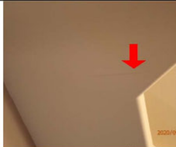
Minor cracks were noted on the second floor ceiling.
