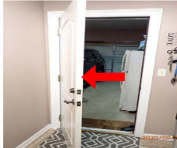
Garage entrance door to the house should be on a self-closing hinge.
