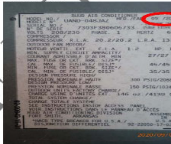
Outside condensing unit MFD: 09-2006
