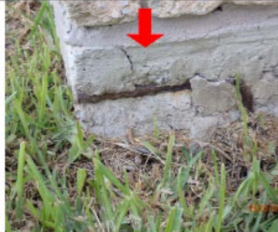
Foundation wall mortar joints show evidence of deterioration.
