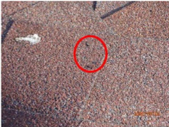
Nail heads are exposed at the ridge.
