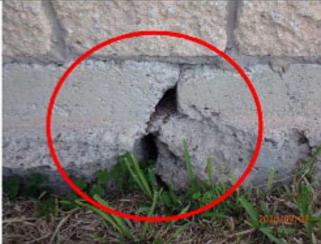
Foundation wall mortar joints show evidence of deterioration.
